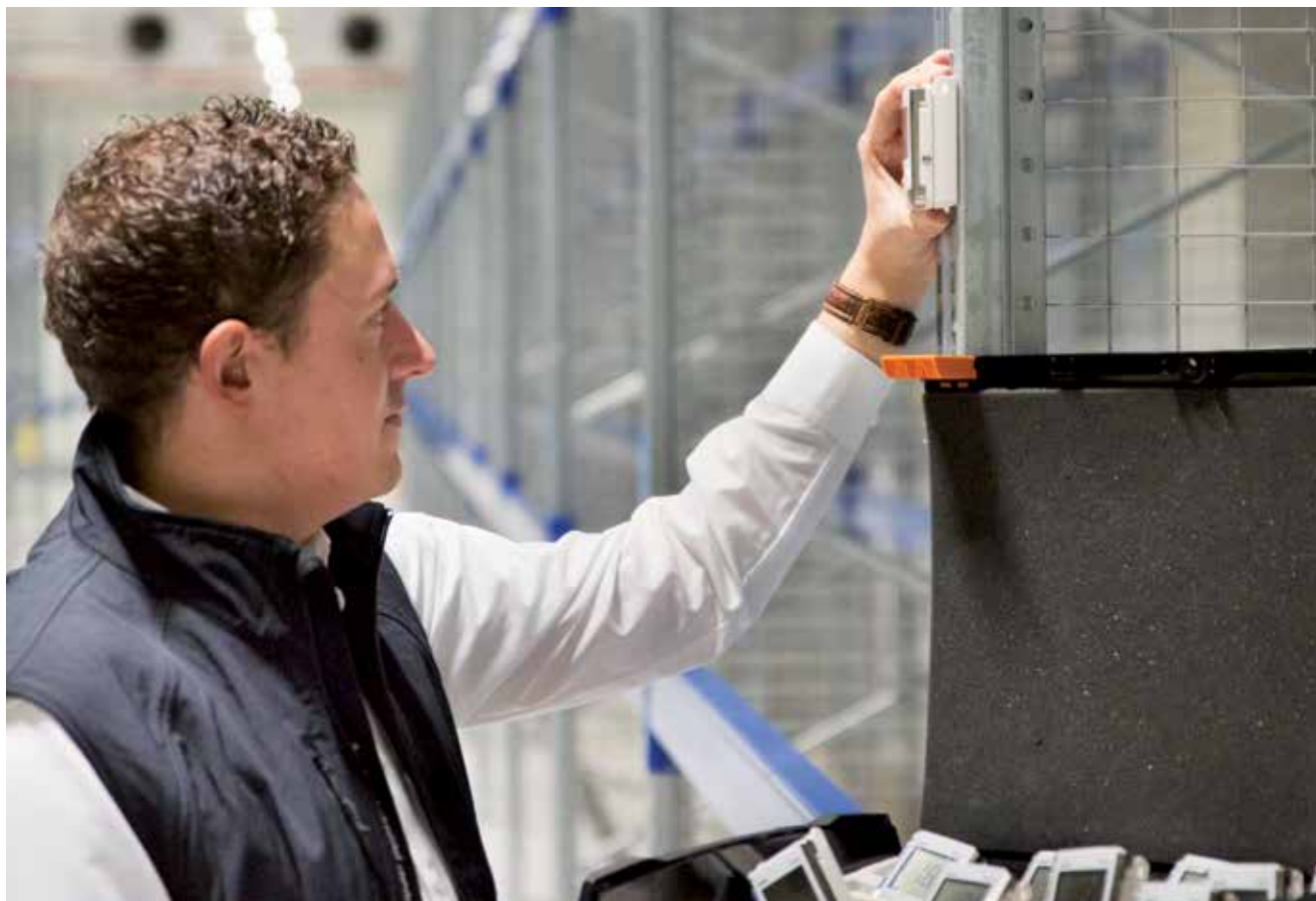
A specialist from Testo Industrial Services installs a data logger testo 175.
