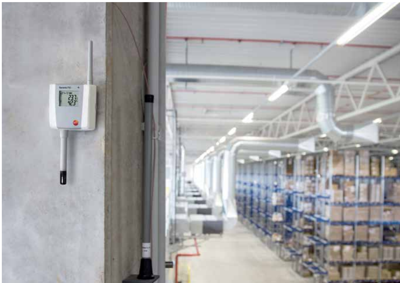
Constant monitoring of temperature and humidity is indispensable in the storage of pharmaceutical goods.
